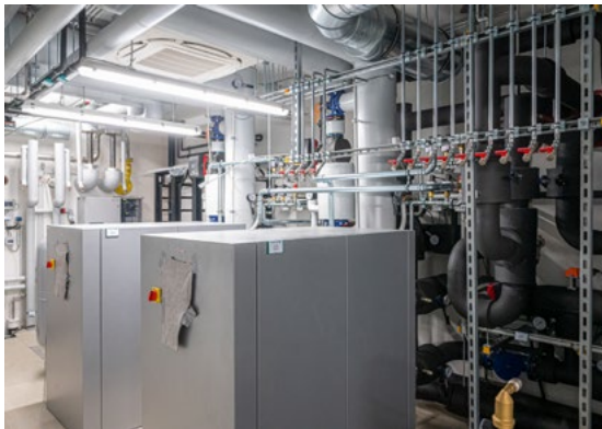
Modern heating systems can be optimized by enabling remote reading.
